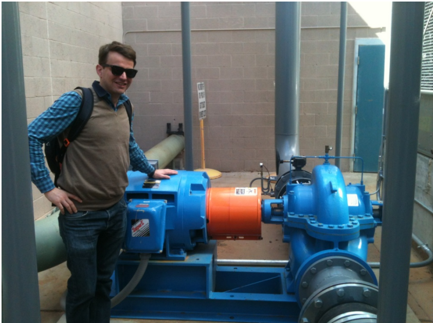
Fig. 3: Heat rejection pump at the world's most powerful solar cooling installation in USA (Source: SOLID)
