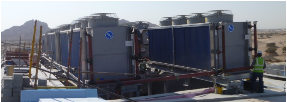
Fig. 2: Heat rejection system for a large solar cooling system in desert environment (Source: SOLID)
